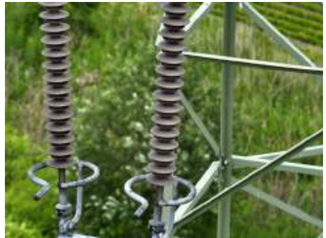
Figure 2. Detailed view of isolators - with usage of hybrid zoom it is possible to accurately inspect the technical condition of the implemented devices.
