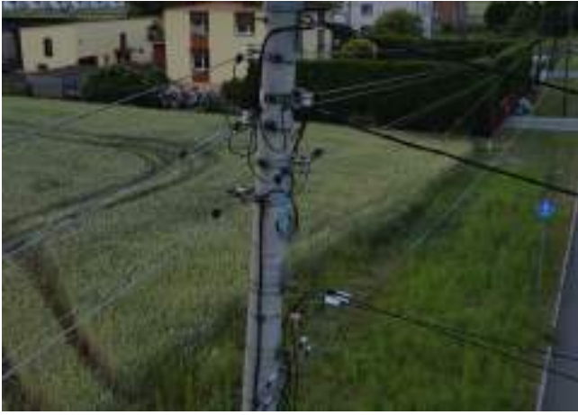
Figure 1. Low voltage power transmission line – the use of UAVs enabled detailed visual inspection, even at the line-congested spots.
