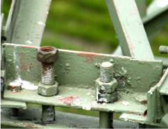
Figure 3. The attachment of the isolator system bracket with an apparent anomaly (unscrewed nut of the attachment clamp). The photo was taken from 8 m using a camera with 16x optical zoom and 200x hybrid zoom.
