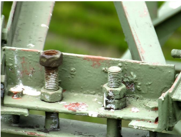
Figure 3. The attachment of the isolator system bracket with an apparent anomaly (unscrewed nut of the attachment clamp). The photo was taken from a distance of 8 m using a camera with 16x optical zoom and 200x hybrid zoom.
