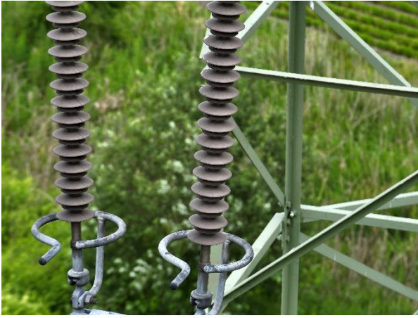
Figure 2. Detailed view of isolators - with the help of hybrid zoom it is possible to accurately inspect the technical condition of the implemented devices.
